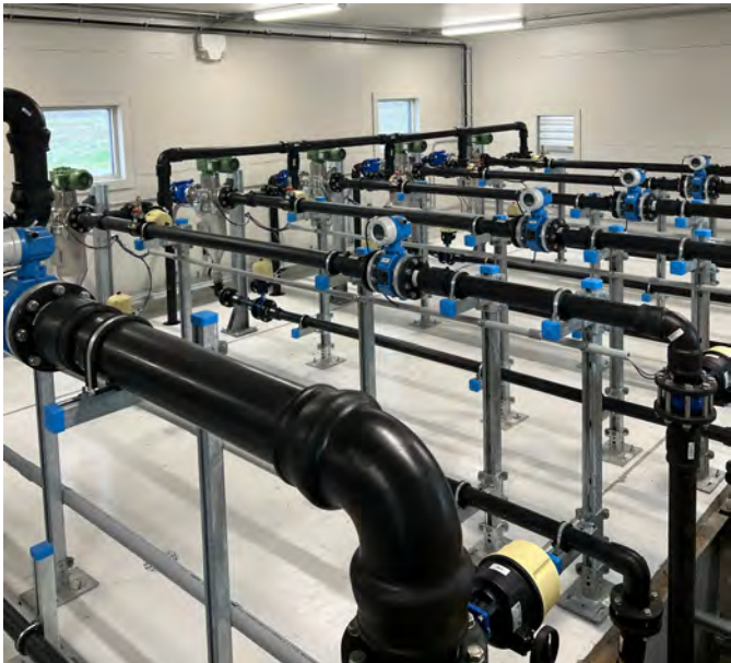
Pump station equipped with all features
